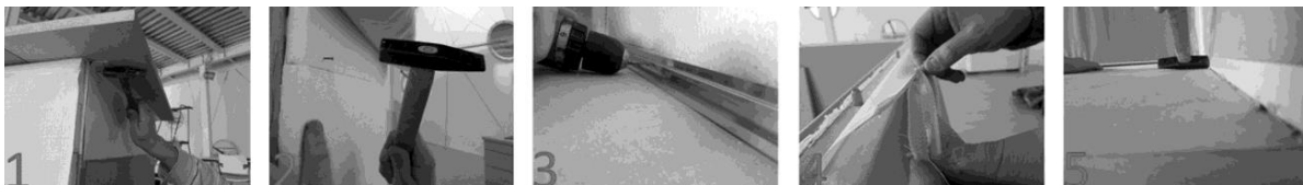
Fig. 2. Sequence of assembly, solution no. 2: 1 - fixing the PVC strip to the wall; 2 - installing the insulation layer in front of the PVC strip; 3 - fixing the lower profile; 4 - connecting the finishing fabric to the PVC strip with a plastic cursor; 5 - fabric fixing at the bottom edge.
