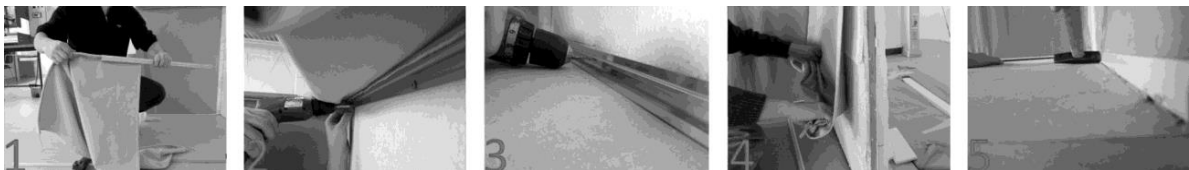
Fig. 1. Sequence of assembly, solution no. 1: 1 - inserting fabric with Keder bar in the upper profile; 2 - fixing the upper profile; 3 - fixing the lower profile; 4 - fabric tensioning; 5 - fabric fixing at the bottom edge.
