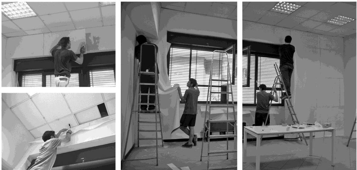
Fig. 4. Test of the insulating wallpaper with the final solution for the tensioning system, July 2015.
